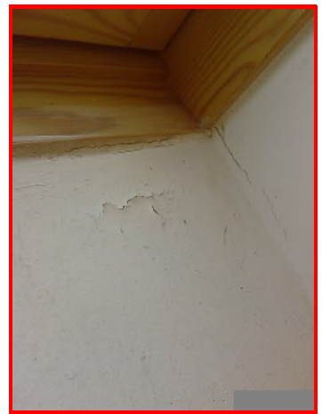
Bathroom Window Window frame/sill - peeling (lightly)
