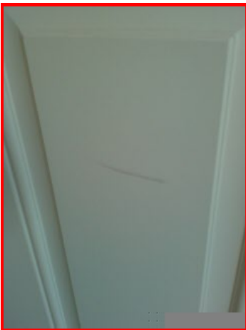
Bedroom 1 Door Door finish - marked (lightly)
