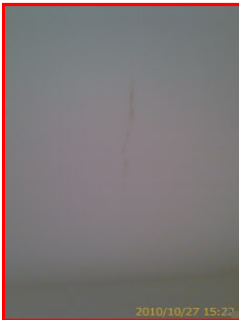
All of Ceiling to Room Ceiling finish - cracked
