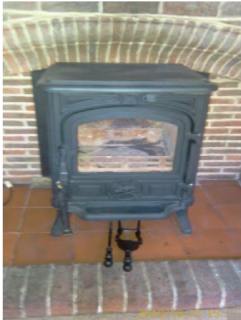
Wood burner and brick fireplace
